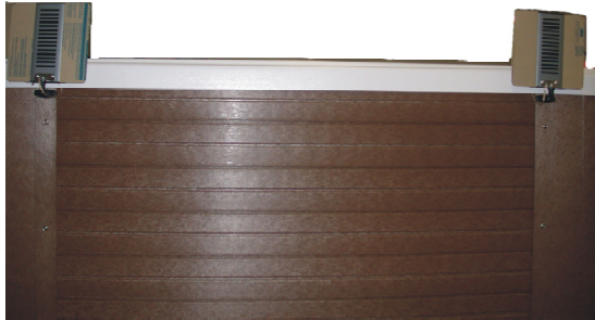
Figure 43. Typical Satellite Speaker Installation
